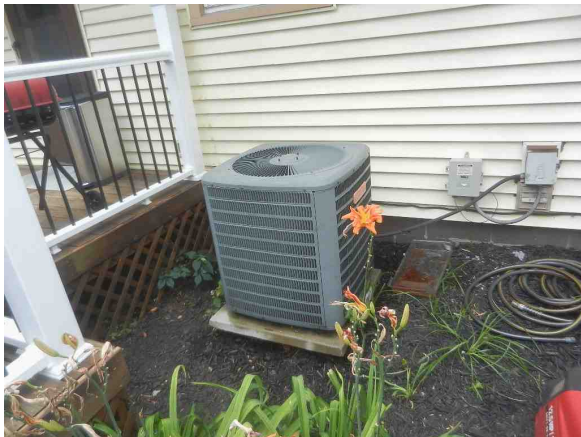
Central air unit
